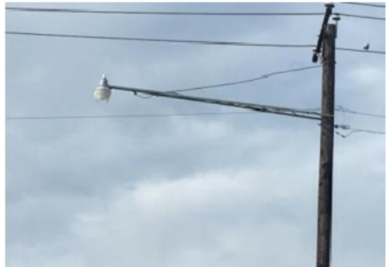
EXISTING STREETLIGHT EXAMPLE
