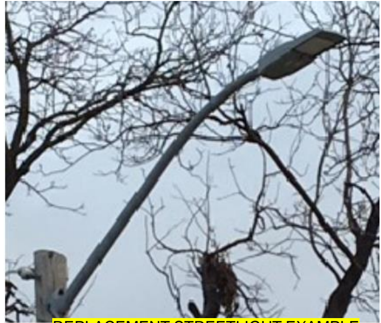
REPLACEMENT STREETLIGHT EXAMPLE
